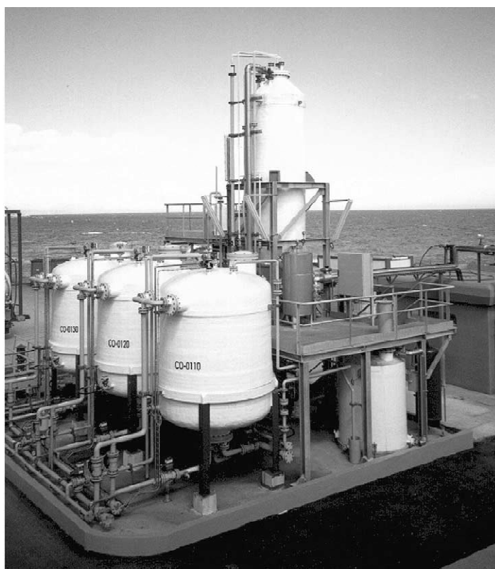
Fig. 1. The Guzina plant chloroform removal unit.
